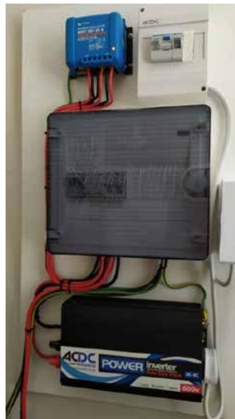
Figure 5. Domestic 600W ESS: PMMT solar charger top left, 230VAC O/L and E/L protection top right, DC DB centre with DC O.C protection for all DC components and surge protection on PV array supply for proximity lightning discharges and the 600W pure sine wave inverter at the bottom. This system is completely off grid supplying all home communications, office and entertainment systems.
