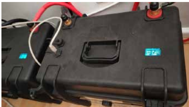
Figure 4. Lithium Fe PO 4kWh ESS with digital battery monitoring system (BMS) with built in digital displays and BMS communication capability for smart charger/inverter systems,
