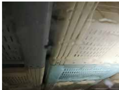
Picture of inside of DCA chamber through port hole window
